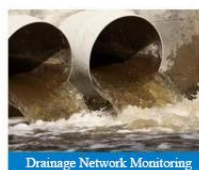
Drainage Network Monitoring
