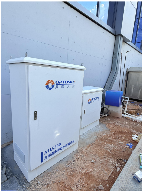
Water Quality Monitoring Application in an Underground Domestic Sewage Well
