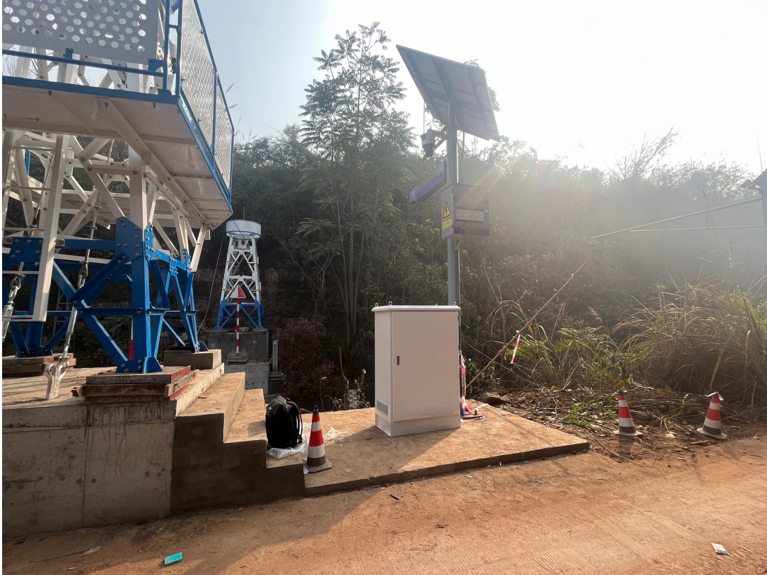
Water Quality Monitoring Application Case in a Reservoir
